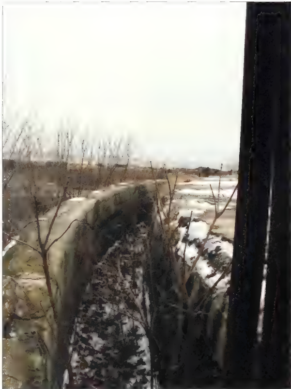
Figure 5.59. View looking east at the chemin de ronde , Battery Potter. Woody vegetation is growing in the chemin de ronde , a designed sentry route located north, south, and east of Battery Potter's superior slope. The vegetation threatens the historic battery's concrete features and surfaces and should be removed. After vegetation removals, the chemin de ronde should be regularly inspected and leaf litter and accumulated debris should be removed to prevent future vegetation growth and to protect the concrete surface (Olmsted Center, January 2009).
